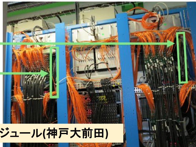
installed in USA15
