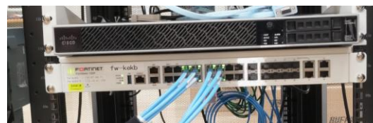
Firewall Fortigate 100F
